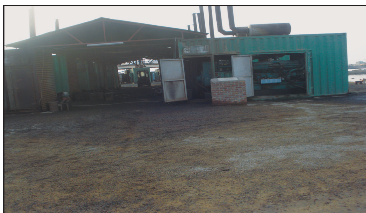
Figure 4.2: Surface contaminated with waste oil from power station-1, a few metres from the sea.
